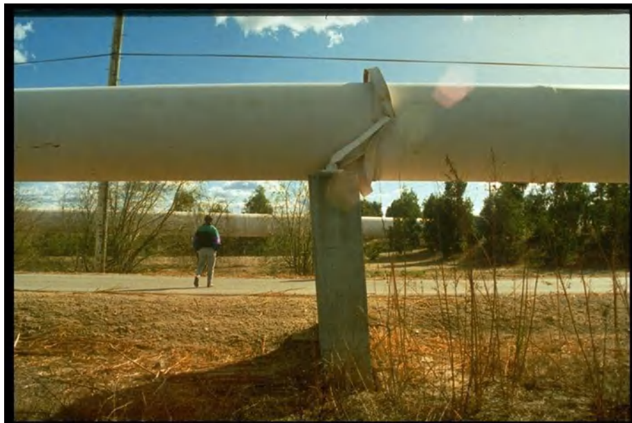
Figure 2-13 : Rupture du support d'une tuyauterie (Northridge, USA, 1994, [R13])
